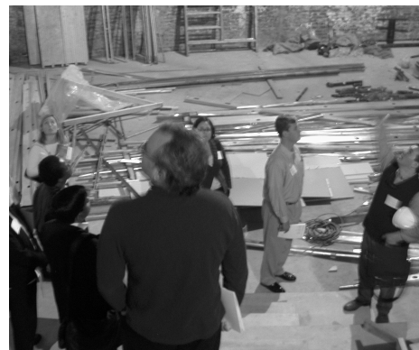
The former Herren's Restaurant is being rehabilitated as a live theater venue. See more pictures of the site in our Industry Council section of www.georgiatruster.org .
